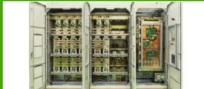
Accelerator power supplies
